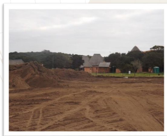
Pictured: The development of El Shaddai school fields by the roads construction company.
